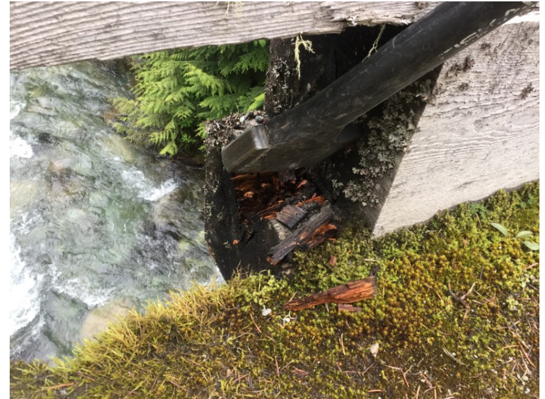
Risers and blocks rotten
